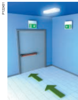
At the safety exits and depending on where the safety signs are installed.
