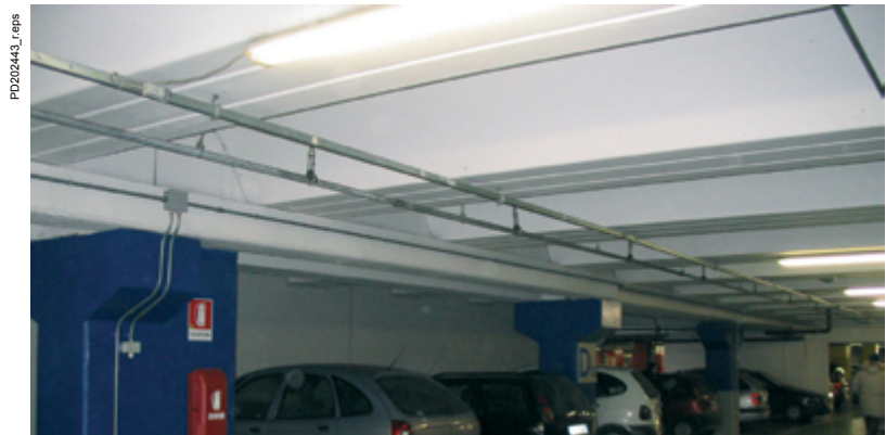
Canalis KBA supplying luminaires nearby sprinklers.
