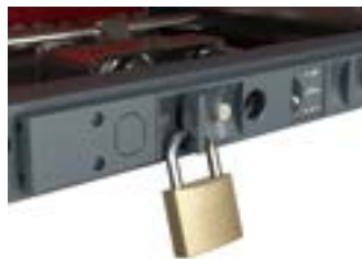
“Disconnected” position locking by padlock.
