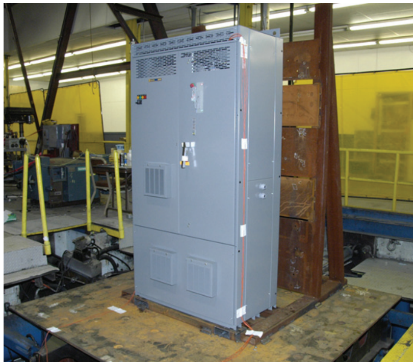
Figure 2: 18-Pulse Device Mounted to Test Stand at Wyle Labs
